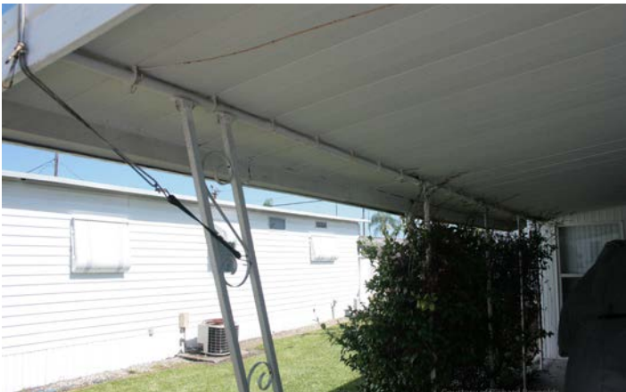
Figure 30. Use of a round beam to provide beam support at eave of carport.
