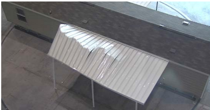
Figure 4. Buckling of pans at mid-span.
