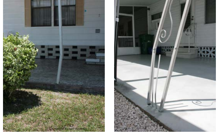
Figure 13. Cracked, fractured, and bent post.
