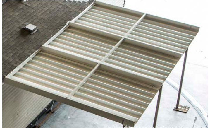
Figure 24. Modified retrofit with two additional 2" x 7" beams so each section of 2" x 4" brace only spanned 8'.
