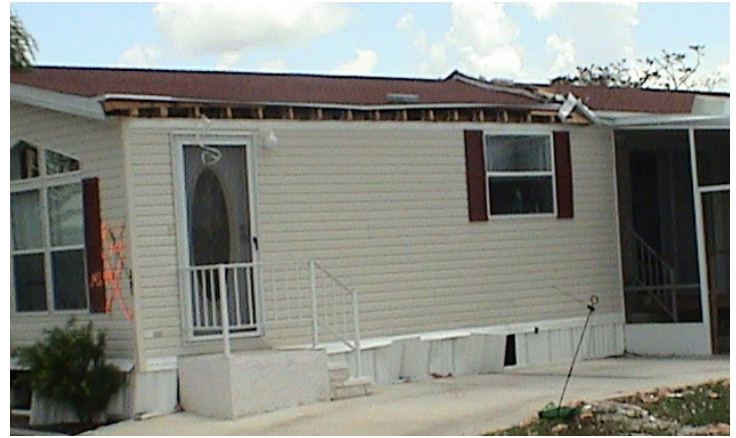
Figure 27. (Above) Typical damage to the eave of a home when a carport roof is blown away during a hurricane. About six square feet of area at the top of the wall was opened allowing entry of wind-driven rain.
