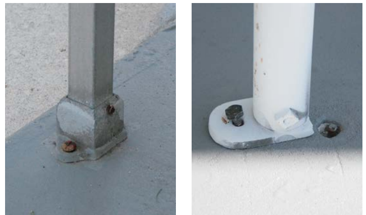
Figure 14. Other examples of poor post connections at base. Cast aluminum bracket (left) and broken bracket with dislodged screw (right). Note inadequate spacing of fasteners from each other.
