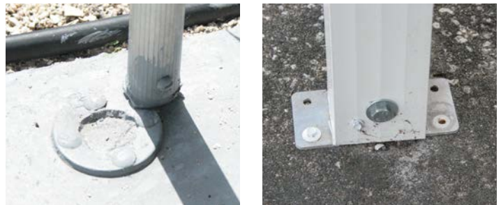
Figure 10. Posts with little or no connection to slab.
