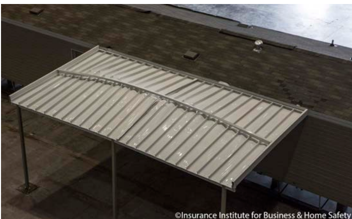
Figure 23. Roof buckled upward when subjected to 80-mph winds.
