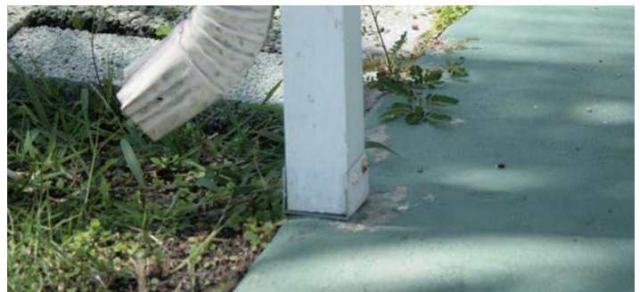
Figure 12. Thin sheet metal and small sheet metal screws are used to anchor post; anchor bolt is hidden under post and much too close to edge of concrete.
