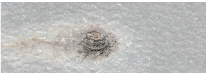
Figure 35. Corrosion around existing fastener without isolating neoprene layered washer.
