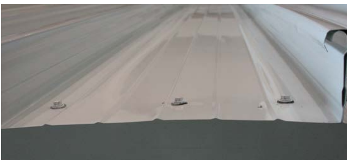
Figure 34. Initiation of panel connection failure at connections using small screws without metal/neoprene combination washers.
