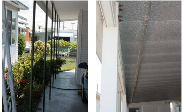
Figure 16. Left image shows typical old support system where pipe posts connect to small thin angle. Right image shows carport with replacement beam and 3" x 3" posts; note severely rusted bolts.
