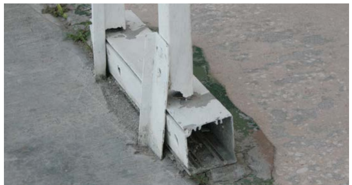
Figure 11. Damaged decorative support with weak repair attempt of connection/support at base.
