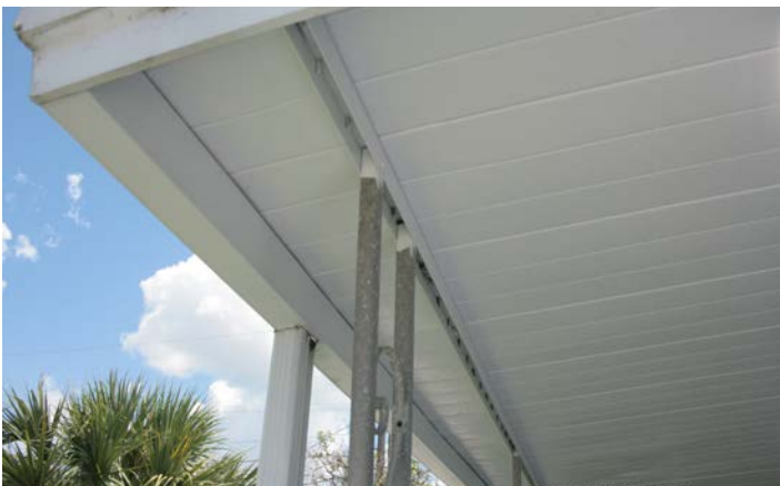
Figure 31. Use of a thin sheet metal-like channel to provide beam support at eave of carport.
