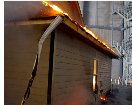
Indirect ignition. Debris in the gutters was ignited by embers.
