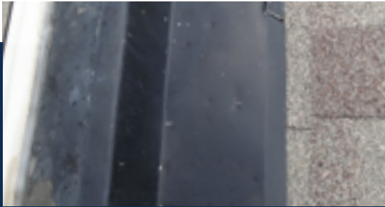
dents in metal flashing
