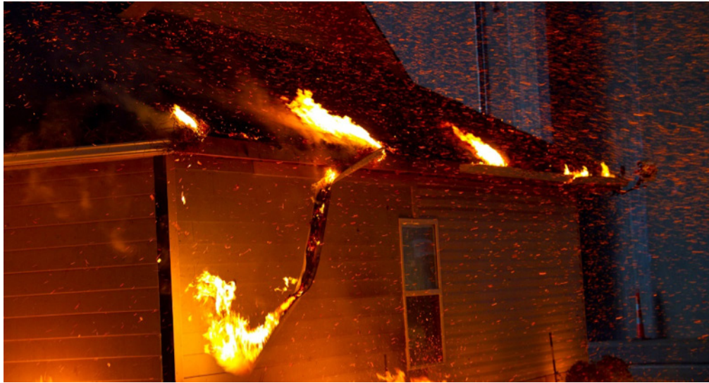
Figure 11. Gutters on fire and melting during an ember attack demonstration in the IBHS large test chamber.
