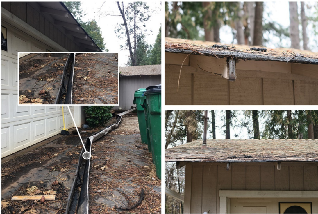
Figure 10. Examples of vulnerability of gutter to ember exposure in the Magnolia community after the Camp Fire.
