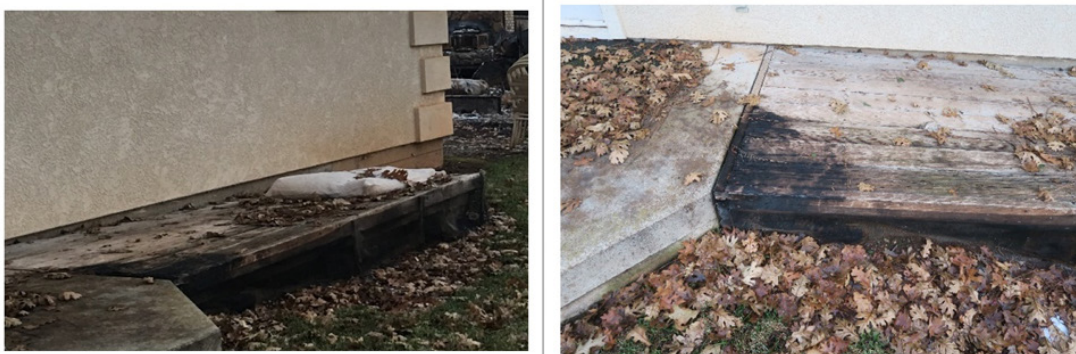
Figure 8. Charred deck and mesh screen from the same home shown in Figure 7.
