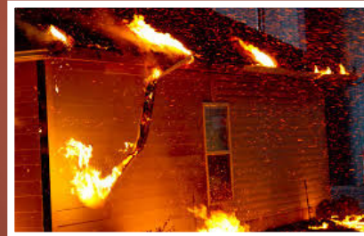
IBHS research shows the risks gutters pose when debris ignites and exposes an exterior wall to a burning plastics fire.
