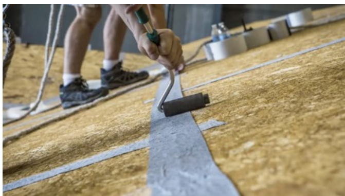
Figure 1. Installing a sealed roof deck system; taping the seams of roof sheathing.
