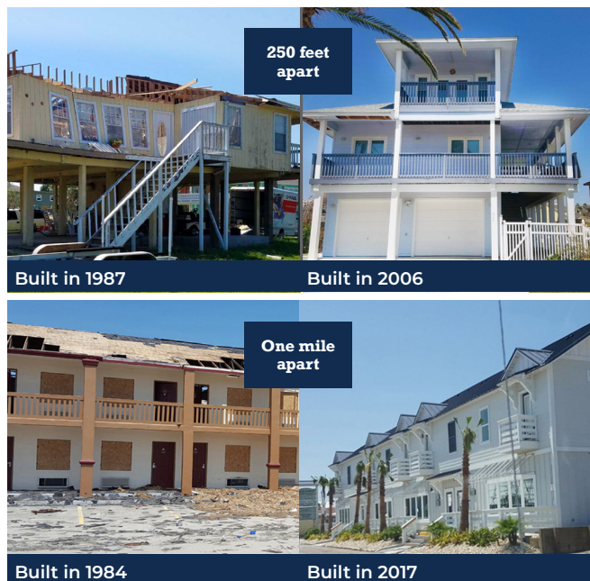
Two examples of damage to older versus newer construction after Hurricane Harvey.
