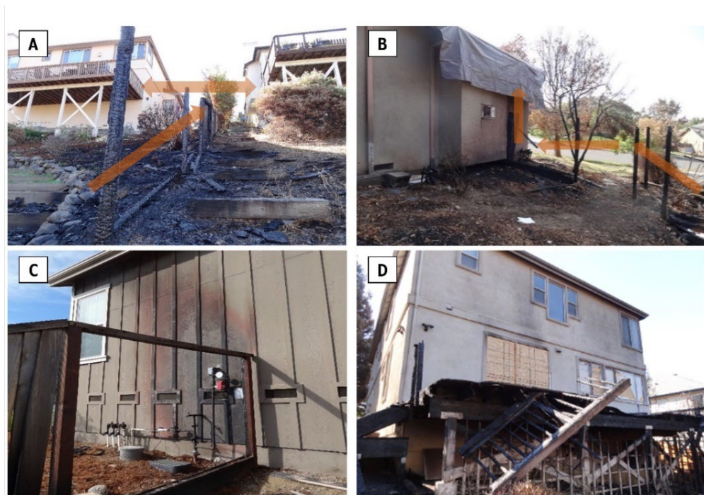
Figure 9: Examples of structural fuel connectivity and the role in damaging the main building in a parcel during the Glass Fire. A combustibile fence (A and B) supported flaming ignition, moving from downhill all the way to the main building, and caused severe damage (C and D). A and B are annotated with arrows representing the estimated direction of fire spread.
